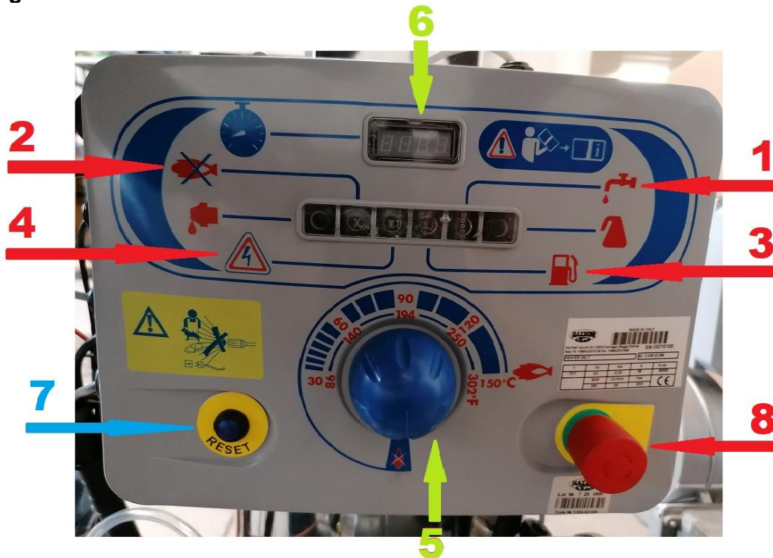
Rev. 1 heater control panel
